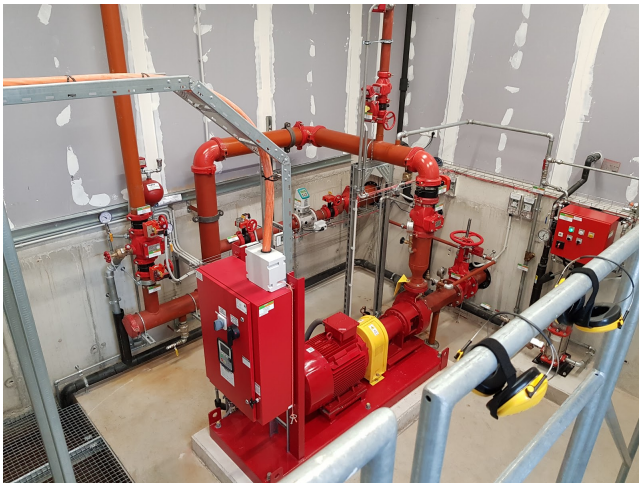
Figure 1: Sprinkler Room with Sprinkler Installation.
