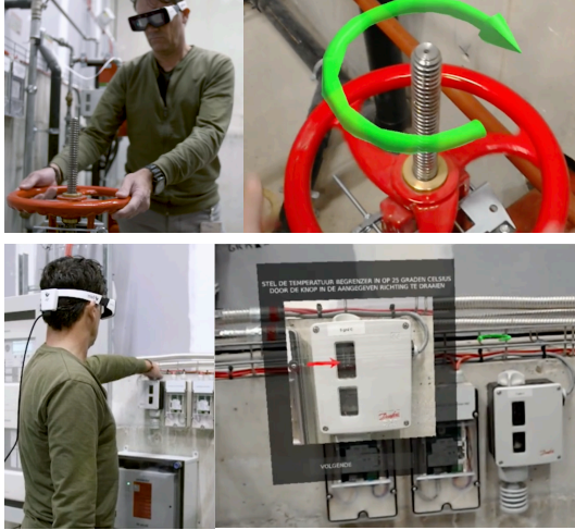
Figure 3: Top panel (right) displays dynamic AR annotations seen through the DSG. Bottom panel (right) displays the required temperature setting on a temperature sensor & dynamic green AR annotation above the button on the far right, © BAM Netherlands [1]
